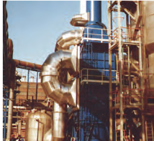
Hot blast generator Umicore, Belgium
